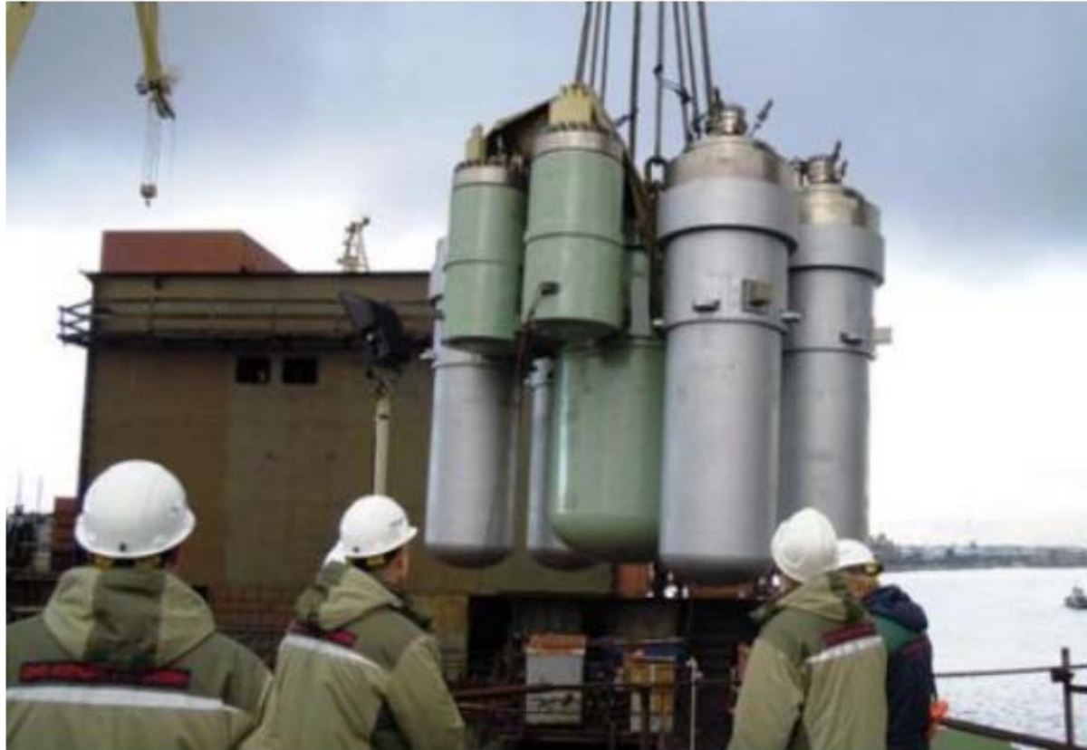
The first steam generating unit - comprising the reactor, steam generators and pressurizer - is lowered into the vessel's reactor compartment (Image: Rosenergoatom)
